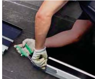
Cut out top leg of inner gable trim to allow for tight, waterproof overlapping.
